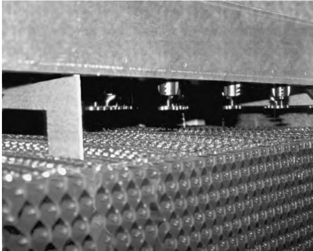
Eliminator air-seal removed showing distribution area above fill
