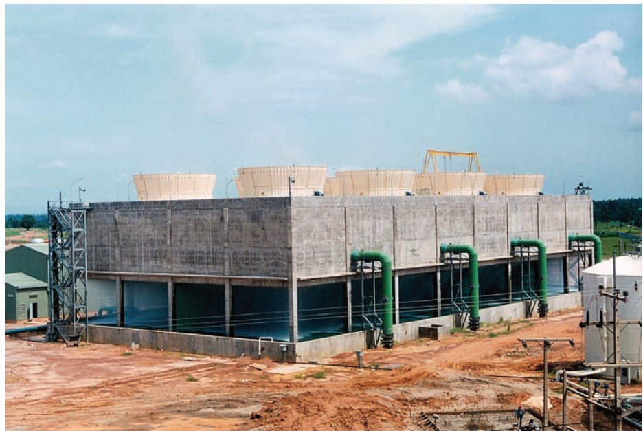
8 Cell Power Station in Thailand
