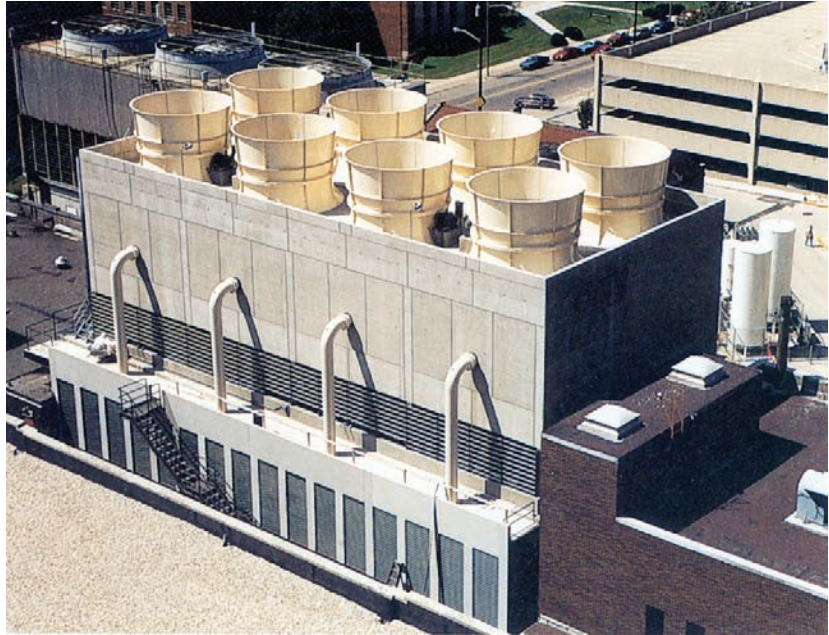
8 Cell Medical Center HVAC system
