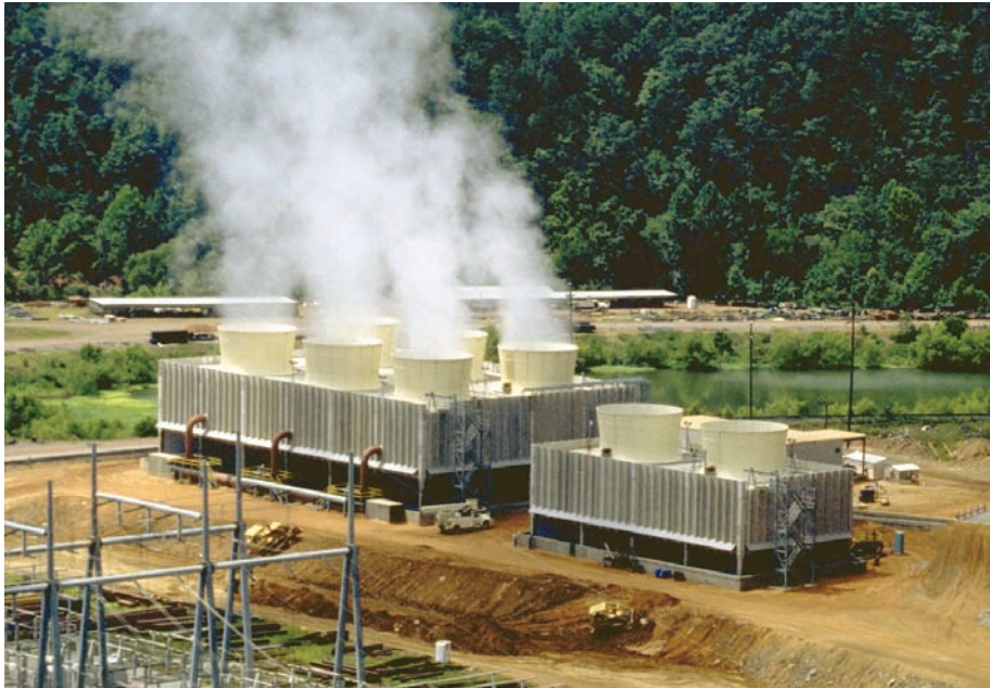
8 Cell Power Station in Alabama
