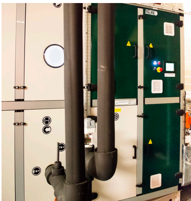
An installed DST Flexisorb dehumidifier in Oasens ice rink ventilation room
