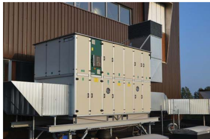
CF-192S installed at yeast factory in Denmark, for spray drying of yeast extract.
