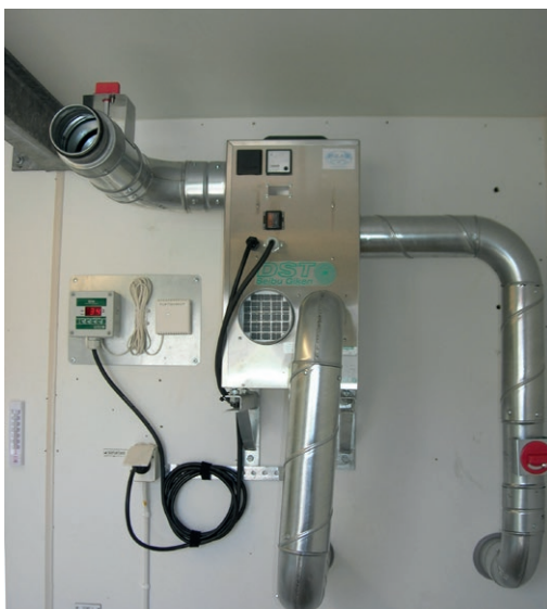
A DR-010B with DST humidistat EH4 controls moisture at a water booster station
